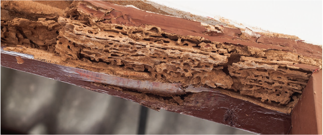
Termite damage to wood
